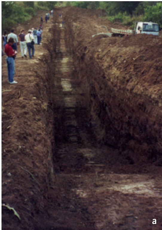
Figure 1: Construction of an underground dam; (a) a trench perpendicular to flow in an alluvial valley is dug down to bedrock; (b) the bottom and wall of the trench is lined with plastic; (c) an extraction well is emplaced in the trench and then the trench is backfilled; (d) salt extracting plants are grown in the alluvium immediately upstream of the dam to reduce salinity build-up – these are harvested and fed to cattle offsite.
